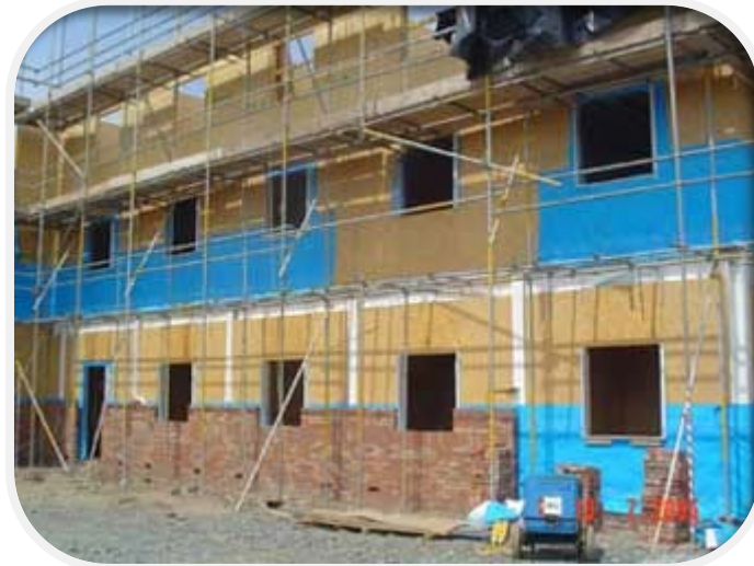
Hemsec SIPs external walls being fitted with breather membrane and external brick skin being installed.
